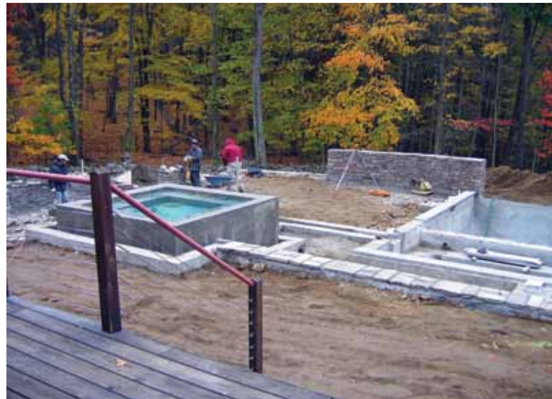
Overflow spa with connecting runnel beyond
